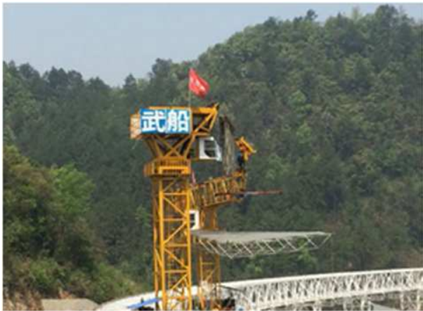
Fig. 8 The second transfer in the air (from transfer truck to cable crane).
