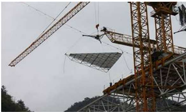
Fig. 7 The first transfer in the air (from crane tower to transfer truck).
